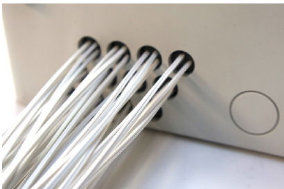
48 ports for Drop Cables
