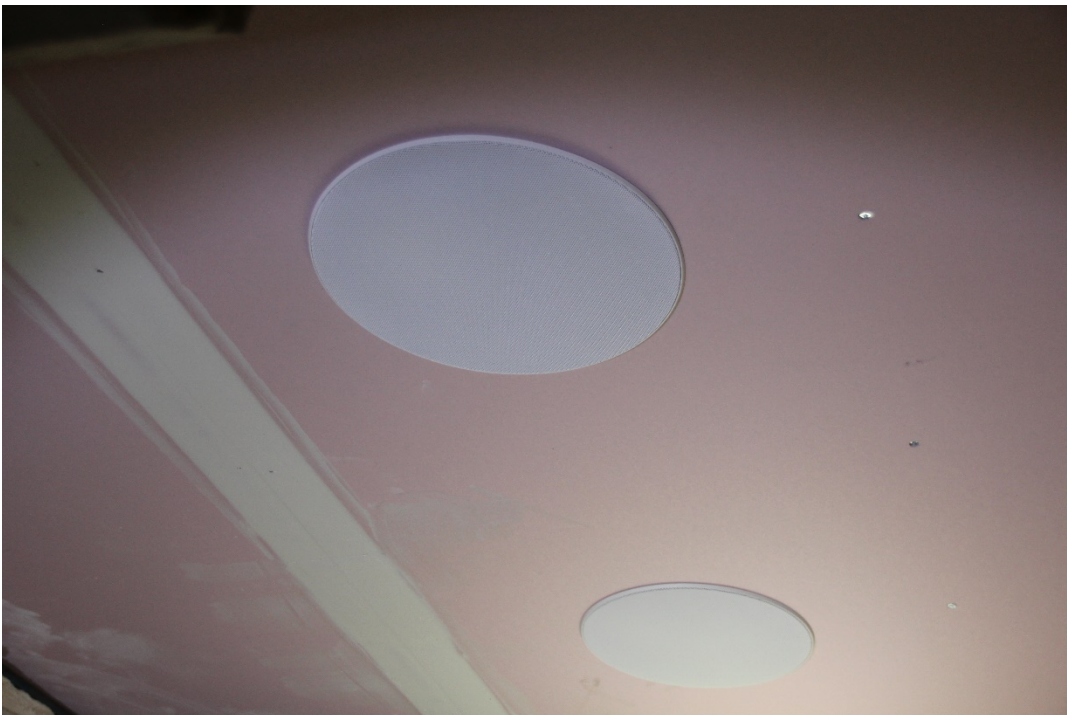
Photo 2 – Before test on exposed side showing the speakers installed into ceiling
